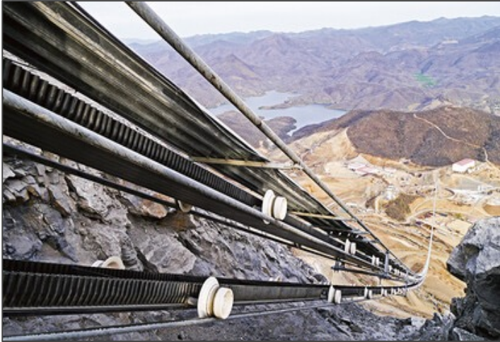
Aerial Rope Conveyor
